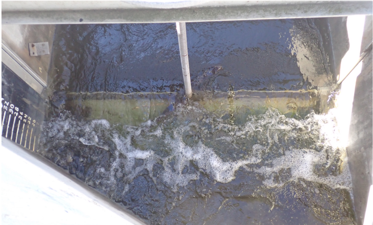
Figure 6. Discharge from the Salinas River Lagoon over the slidegate into the OSR on October 17, 2023.
